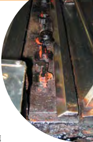
Unacceptable standard of cleanliness and poor maintenance of cooking equipment
