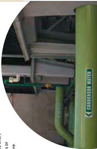
Legionella grows in pipe-work connected to cooling towers
