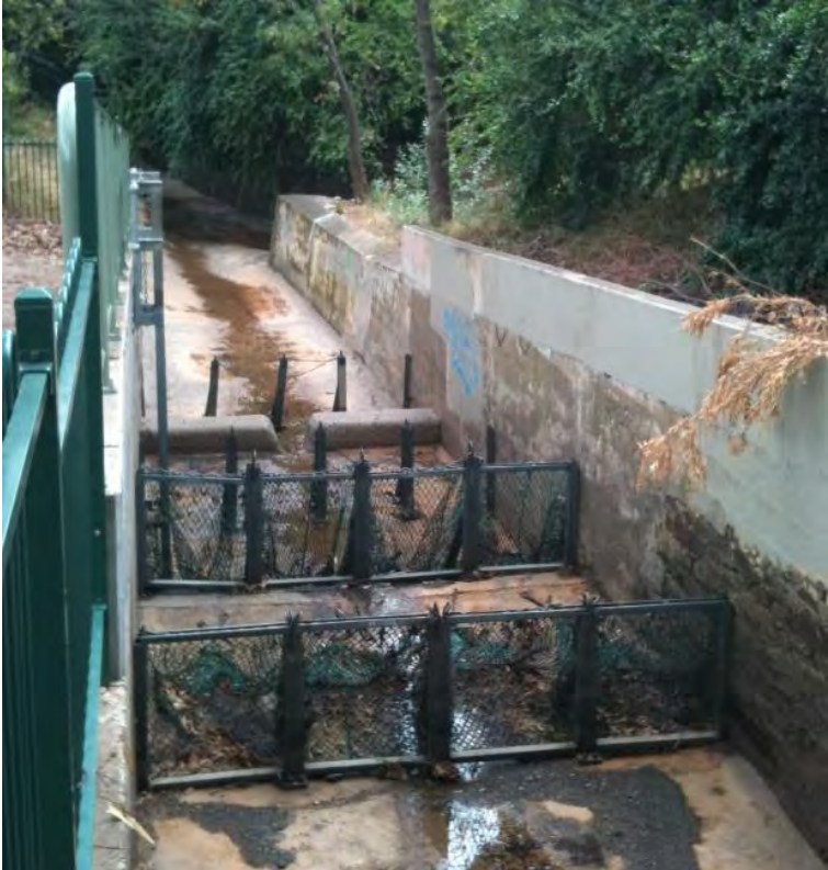
Glen Osmond Creek, Simpson Parade trash racks
