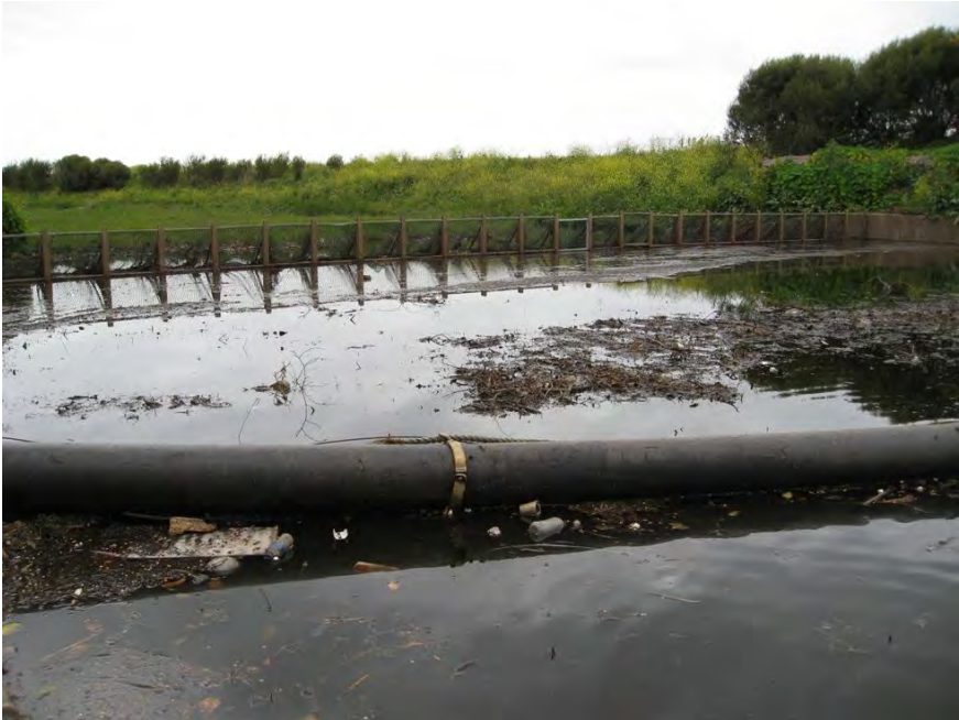
Brown Hill Creek, Watson Avenue trash rack, floating boom and sediment basin
