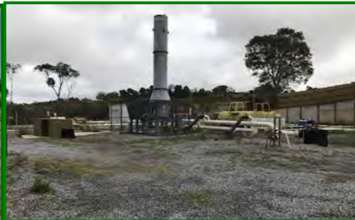
The LoCal flare installed and operating at the Highbury landfill
