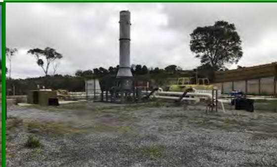
The new LoCal flare installed and operating at the Highbury landfill
